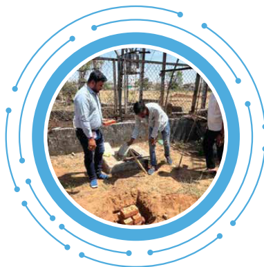
TN-119 Substation Project- Pratapnagar, Jaipur (Government)
