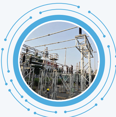
400 kV & 66 kV CIS Substation, Bhogat (Dwarka)
