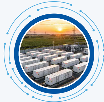
Battery Energy Storage System Project 65 MW/130 MWh-Gujarat
