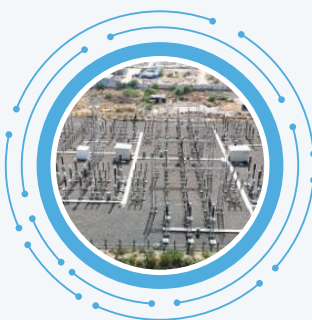
66 kV Power arrangement at GIDC saykha (Private)
